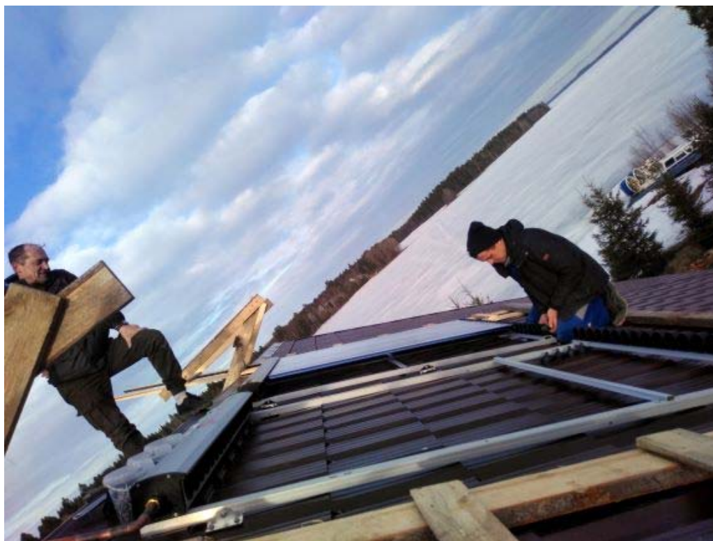
Solar heated water in Kuganavolok Project: Green solution for Nature protected area
